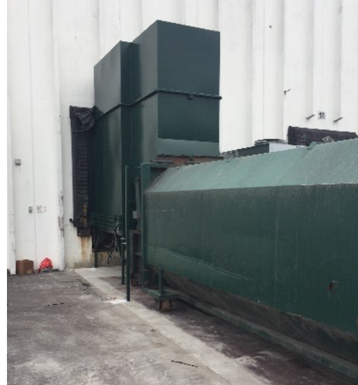
Newly installed Organic Waste Compactor at our Alsip Bakery.
